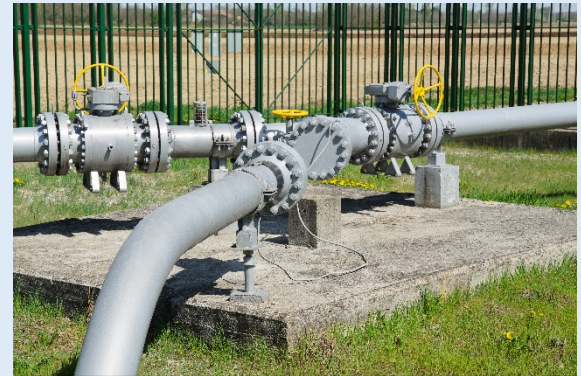
Gas Pump Station
